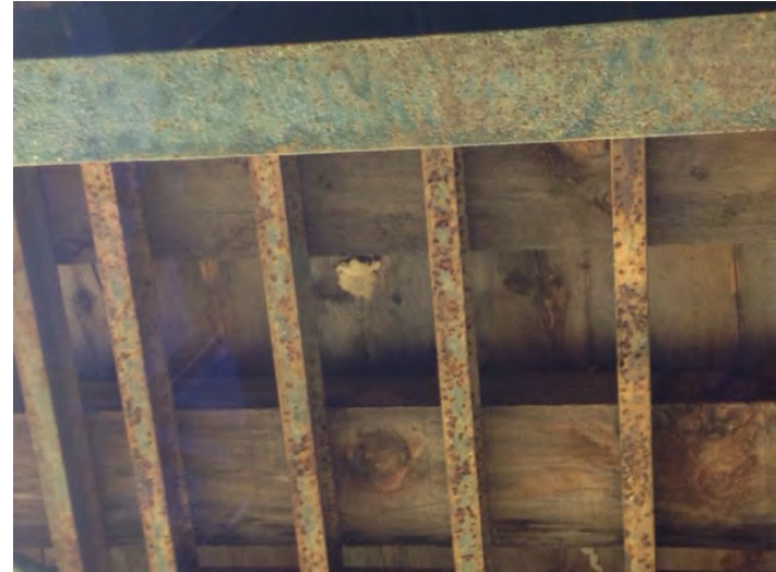
decking starting to rot
