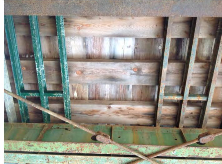
missing steel stringers in 2 separate locations , 20 feet total
