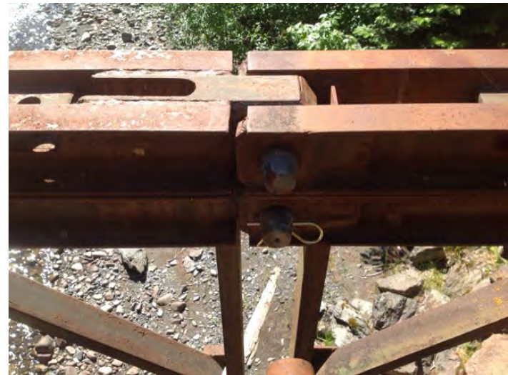
53 missing cotter pins on top 3 missing cotter pins on bearing 2 missing cotter pins on bottom
