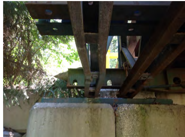
damage to outside panel , right abutment
